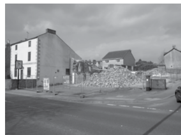
The site of the Weaver on the Butts after demolition in 2013 – but with the inn sign still in situ.
