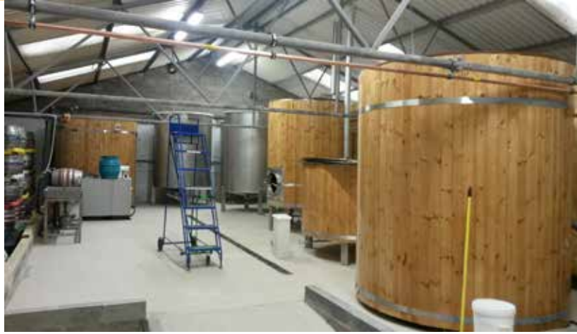
The new Dawkins brewery installation
